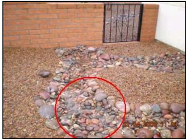
2.4 Picture 2 water ponding present
