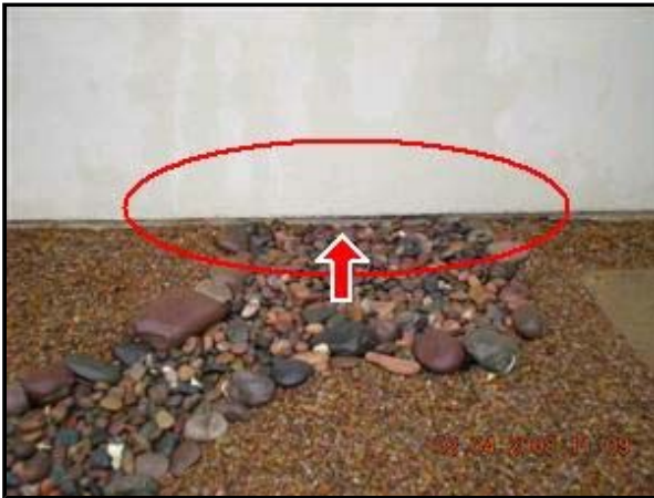
2.4 Picture 1 signs of water intrusion
