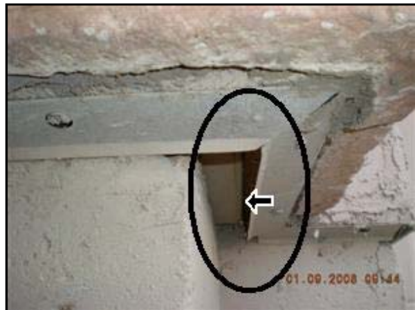
2.0 Picture 2 wood exposed beneath stucco weep screed.
